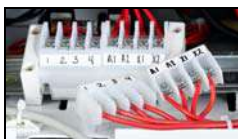
Control Terminal Block
