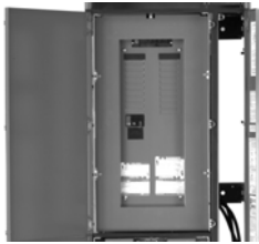
Distribution Panelboard in an MCC
