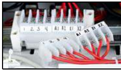
Control Terminal Block
